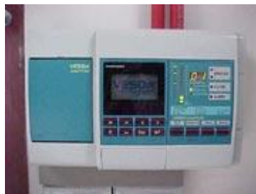
Early warning smoke detection unit
