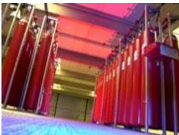
Fire extinguishing equipment
